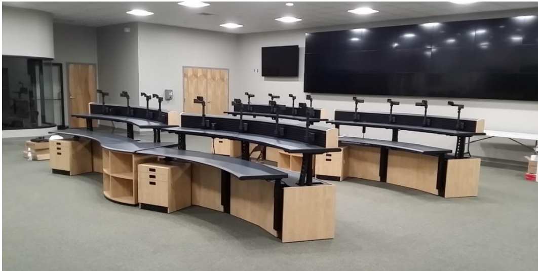
Figure 2-6: District Three TMC Operator Stations
